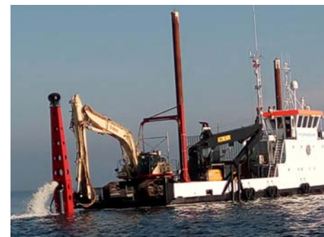
FIGURE 14 Investigation and removal by remote operating device (ROD).
