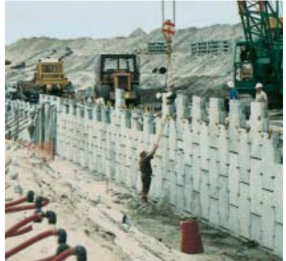
Figure 7. The sea wall structure consists of concrete panels which are built at a rate of 25 to 30 metres per day, thus keeping pace with dredging.
