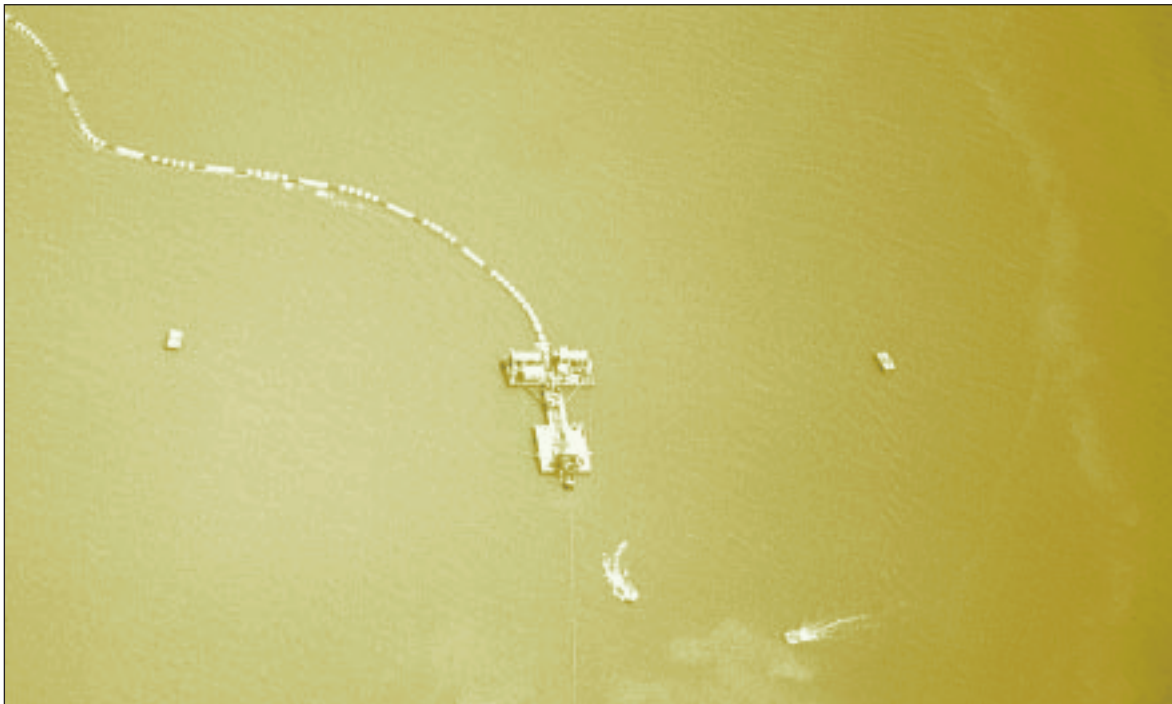
Figure 4. The Willem Bever at work with auger in a box. Specially designed and constructed dredger heads may reduce the turbidity generation substantially. Turbidity clouds seen here in the lower righthand corner are caused by a multicat and the traffic of a working vessel, not by the dredger.
