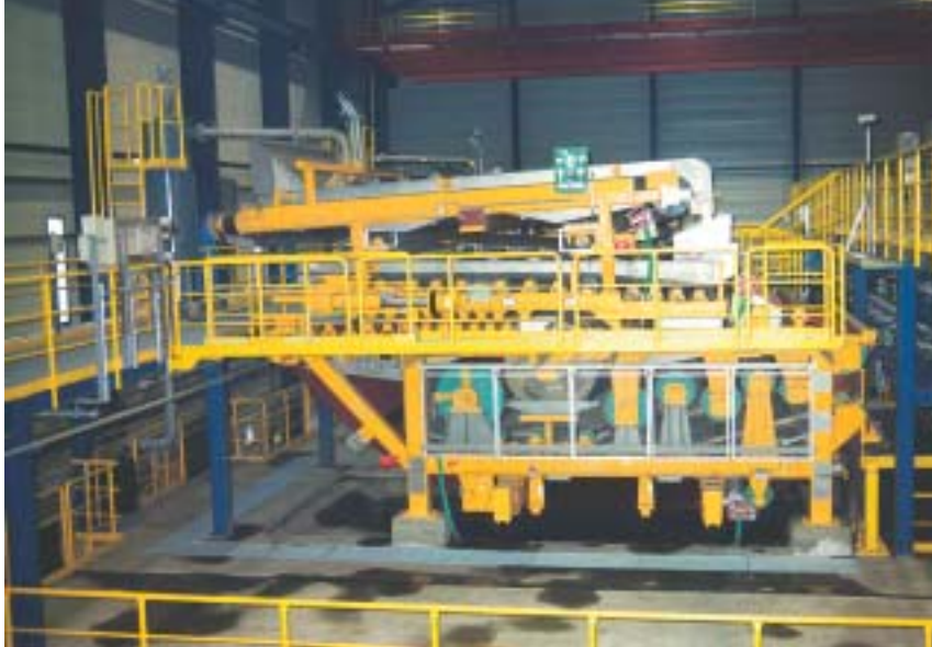
Figure 9. METHA plant: Filter belt presses.
