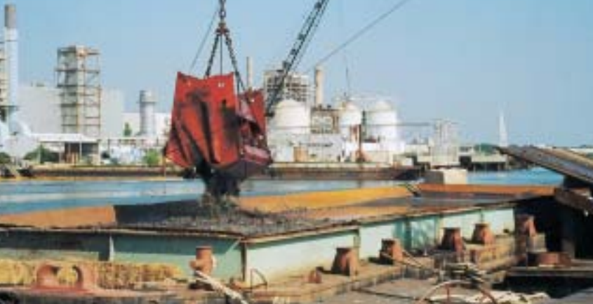
Figure 1. The environmental bucket releasing sediment into the holding barge during July 2004 dredging operations in Jacksonville, Florida.
