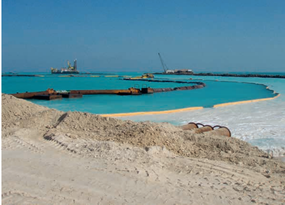
Figure 10. A hanging silt screen at a dredging project in the Arabian Gulf at a reclamation discharge was applied successfully in combination with a breakwater and minimal current velocity.
