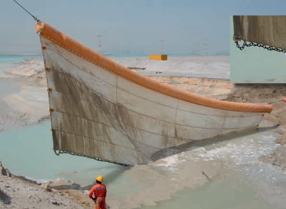
Figure 9. At Saadiyat Island, Abu Dhabi the silt screen did not function in the run-off channel as the current velocity measured exceeded the permitted velocity for the screen, even though weighted down. Current patterns formed around the screen causing fast and turbid flows. Further use of silt screens therefore was suspended. Insert, the ballast chain used to weigh the silt screen down (Taelman, 2009).
