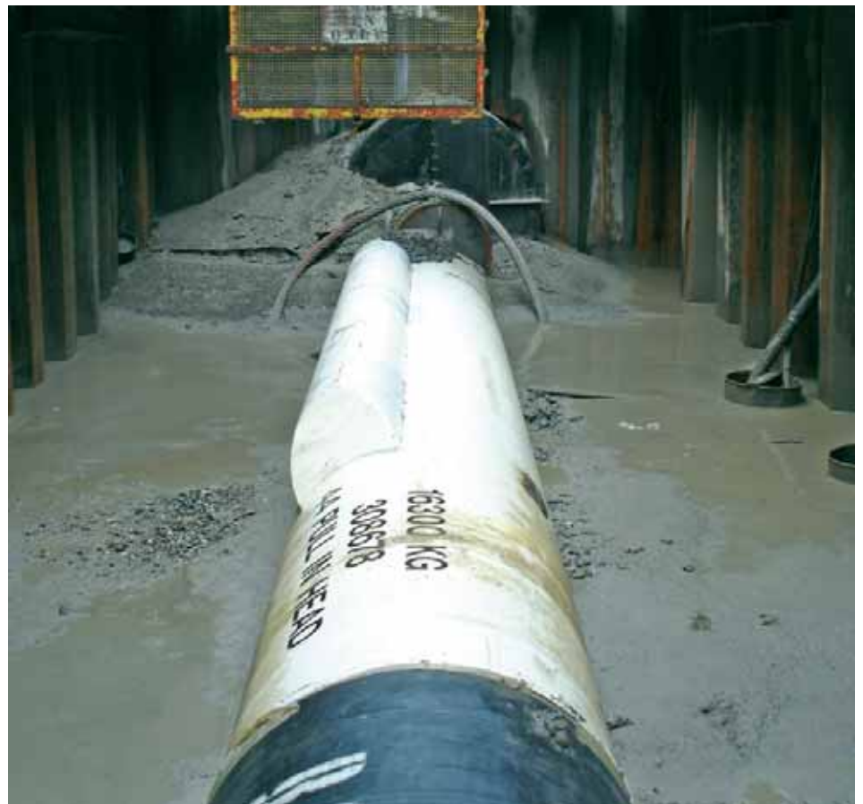
Figure 16. The tie-in between the onshore and offshore pipeline sections was executed at 13 m below low water level.
