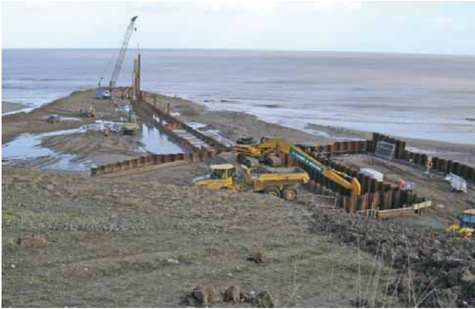
Figure 7. A sheet piled cofferdam was installed by land based equipment working at low tides from a specially constructed causeway.
