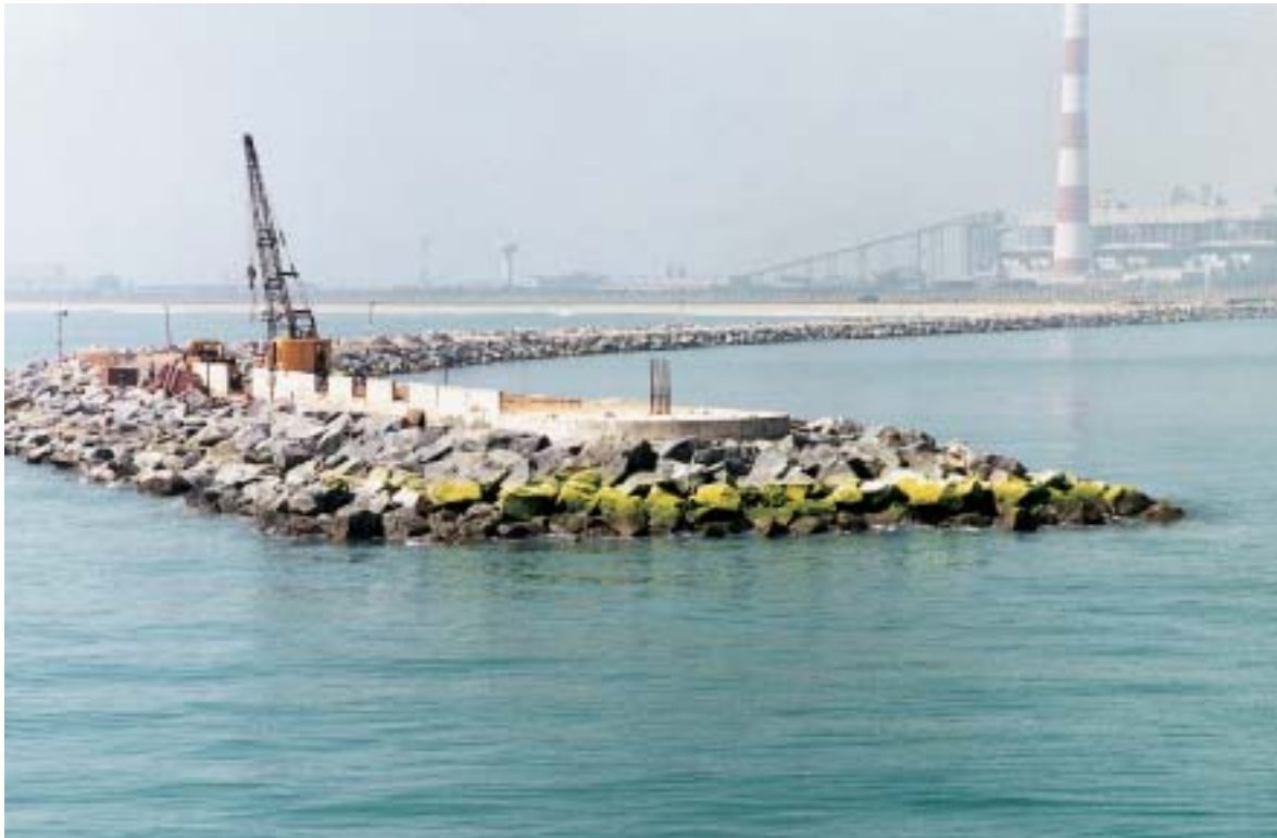
Figure 7. The placing of in situ concrete slab and wave wall at the South Breakwater under construction.
