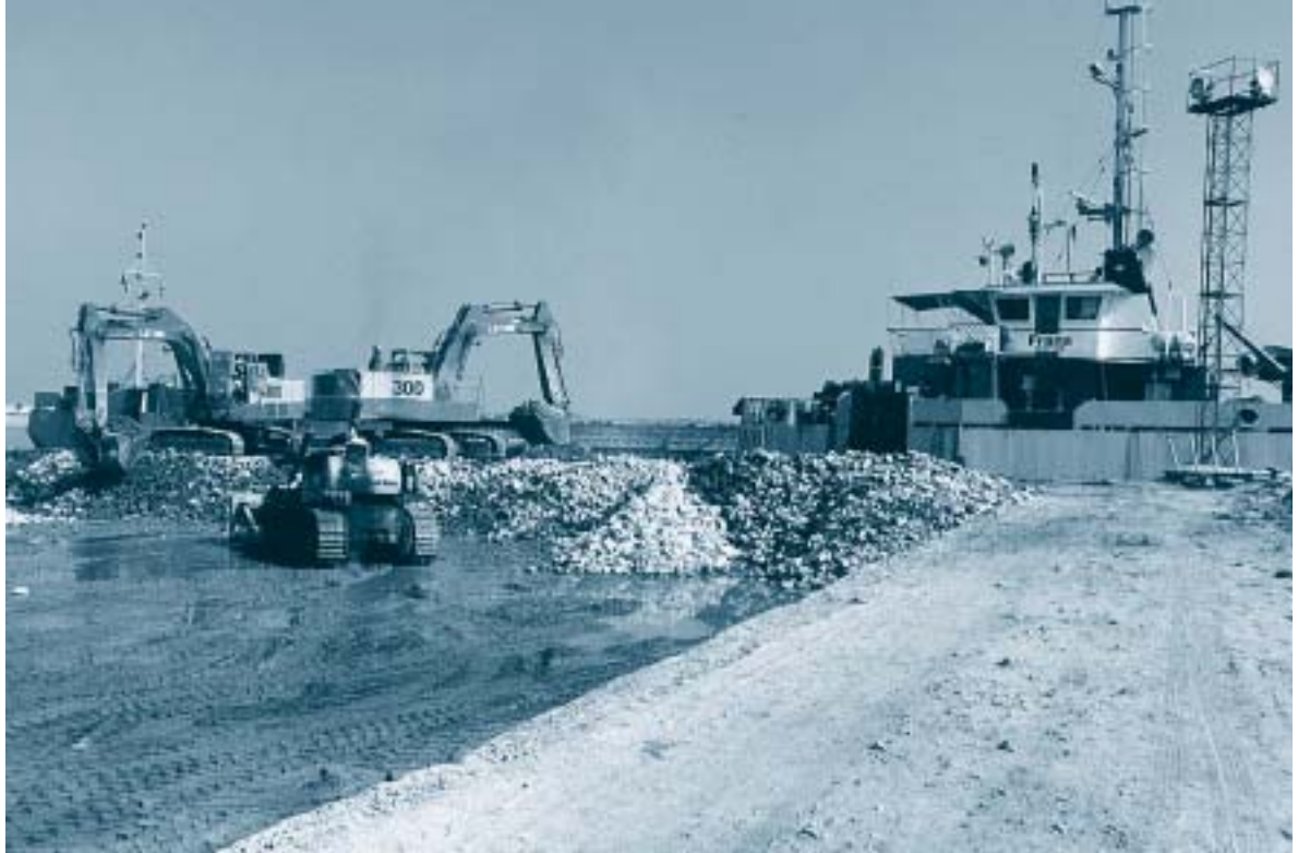
Figure 3. The side stone dumping vessel Frans being loaded at the temporary work harbour.
