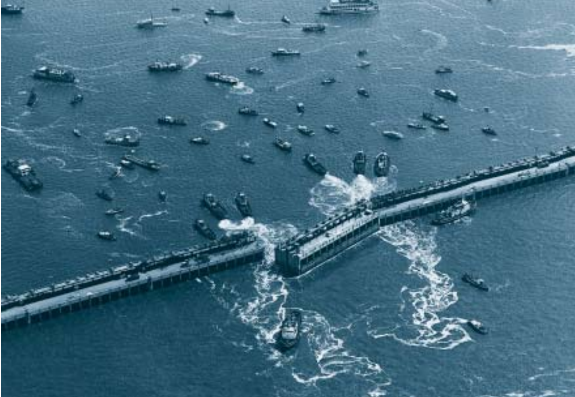
Figure 9. One of the spin-offs of the Delta Project: discharge caissons at the Oosterschelde, being built in 1976.
