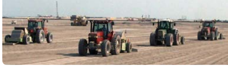
Left, compaction is being carried out with bulldozers in front of the discharge pipe. Right, HEIC is done by impact rollers equipped with modules weighing upwards of 8 tonnes pulled over the new land by tractors.
