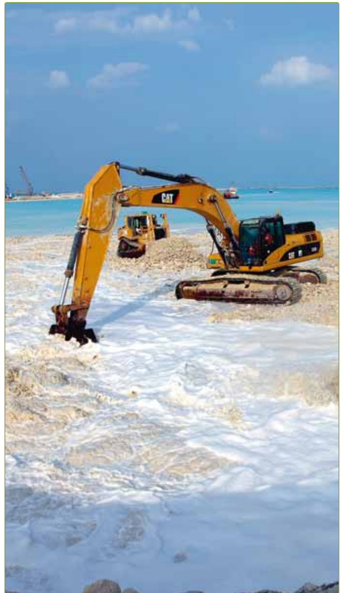
The new Khalifa Port and Industrial Zone (KPIZ), Abu Dhabi was a large-scale design, that included the relocation of Port Zayed from central Abu Dhabi to Al Taweelah.
